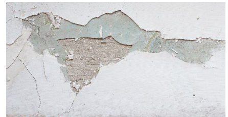
Cracked and flaking paint on a wall
