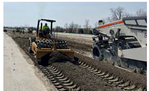
Stabilizing the subgrade under pavement layers can accelerate construction and provide longer-term pavement sustainability.
