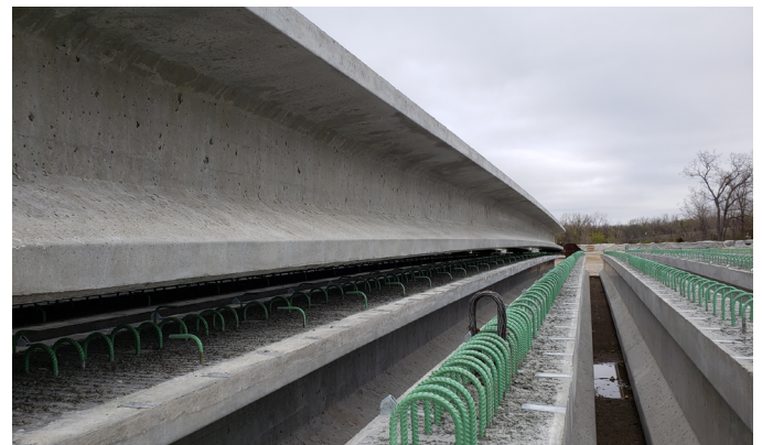
Prestressed concrete beams stored in a fabricator's yard display a slightly arched shape, or camber.
