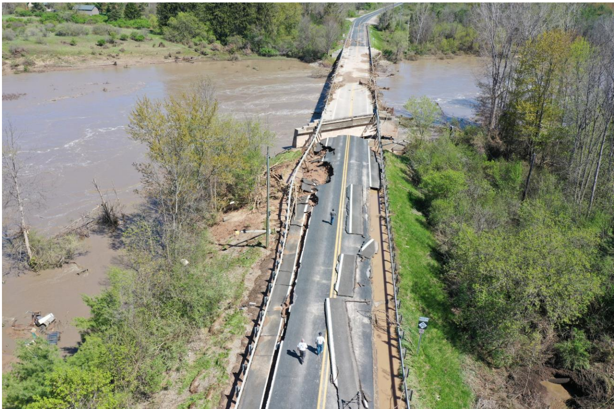
Figure 4. Roadway Flooding in Midland County, Michigan
