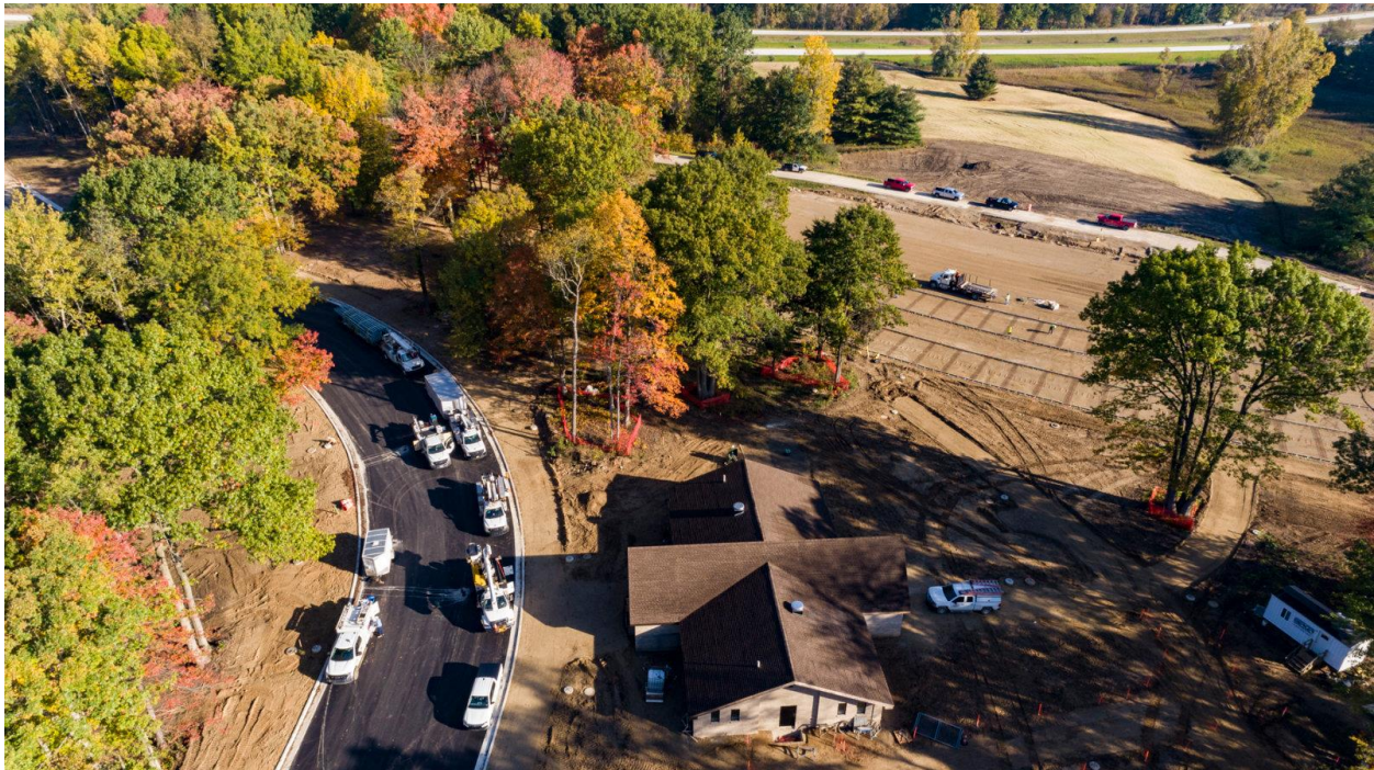
Image caption: Image showing reconstruction of the Five Lakes Rest Area in Lapeer County in September 2023.
