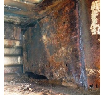
Condition State 4 (Corrosion)
