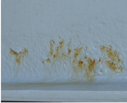
Condition State 2 (Corrosion)
