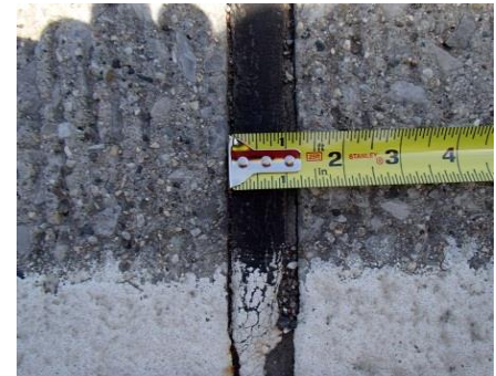
Condition State 4 (PRJ)
