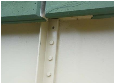
Condition State 2 (Connections)
