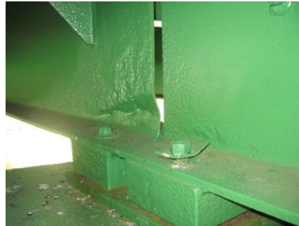
Condition State 3 Deterioration
