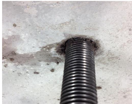
Condition State 3 (Vertical Anchor)
