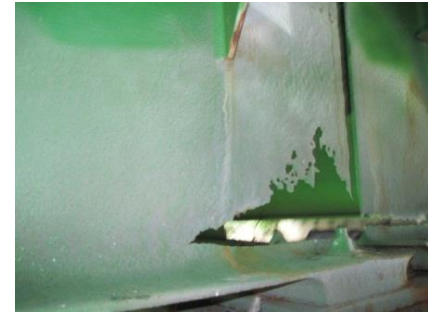
Condition State 4 Deterioration
