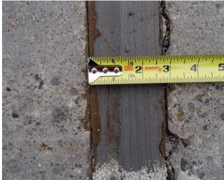
Condition State 2 (PRJ)
