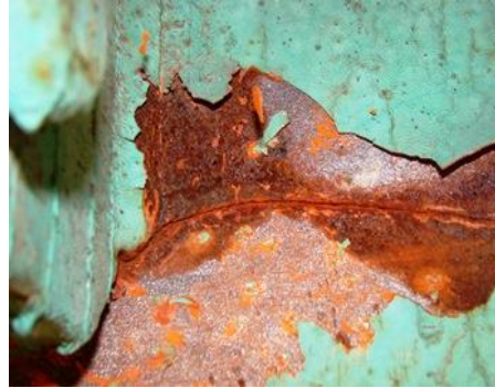
Condition State 3 (Cracking/Fatigue)
