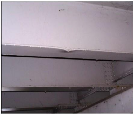
Condition State 2 (Damage)
