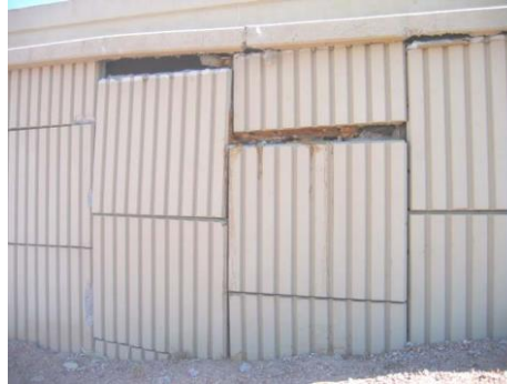
Condition State 4 (Joint Spacing)
