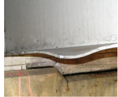
Condition State 4 Beam End Contact
