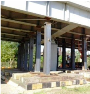
Condition State 2 (Temp Supports)
