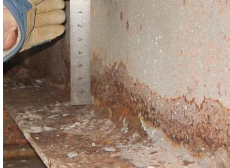
Condition State 3 (Corrosion)
