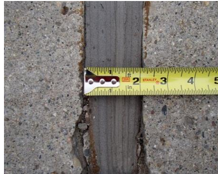
Condition State 3 (PRJ)
