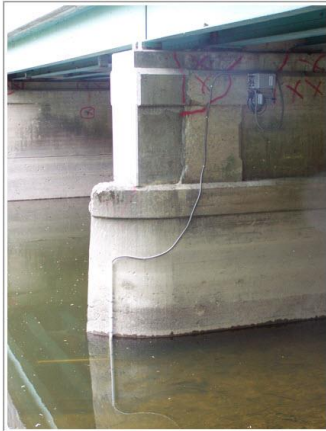
Scour Monitoring Device
