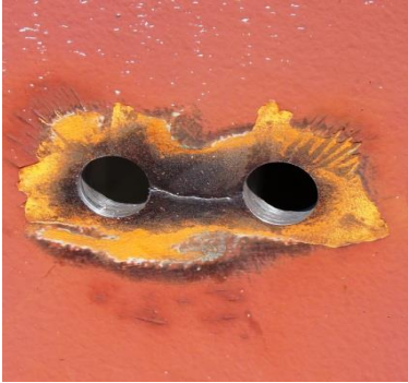
Condition State 2 (Cracking/Fatigue)
