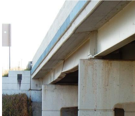
Condition State 3 (Damage)
