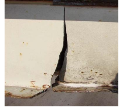
Condition State 4 (Cracking/Fatigue)
