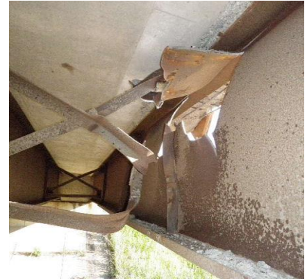
Condition State 4 (Damage)
