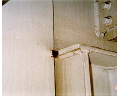
Condition State 3 Beam End Contact
