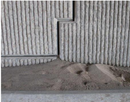
Condition State 3 (Loss of Backfill)
