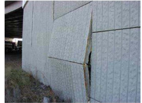
Condition State 4 (Panel Bowing)
