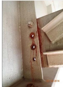
Condition State 3 (Connections)
