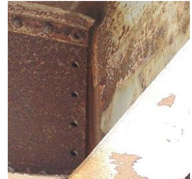
Condition State 4 (Connections)
