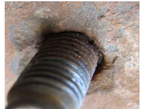
Condition State 4 (Vertical Anchor)
