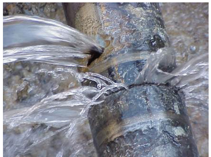
Aging infrastructure like this leaky pipeline contributes to system losses and unrecovered cost for municipalities.
